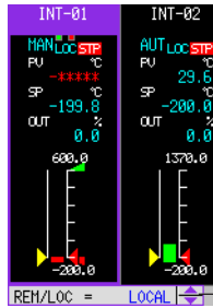
Window for switching between remote and local
